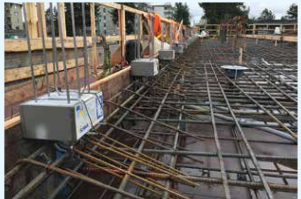
Figure 7. Structural thermal breaks positioned against wooden parapet forms are tied into rooftop reinforcement before casting in concrete.
