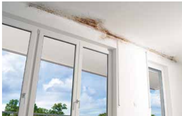
Figure 2. Condensation on the chilled interior side of uninsulated penetrations supports the growth of mold, which can become airborne years before spreading to visible wall and ceiling surfaces.
