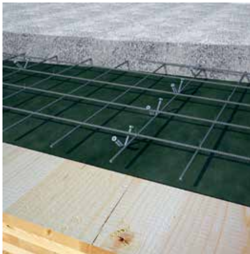
Figure 5. Timber-concrete composite floors made using Rothoblaas CTC timber fasteners. Courtesy of Rothoblaas.
