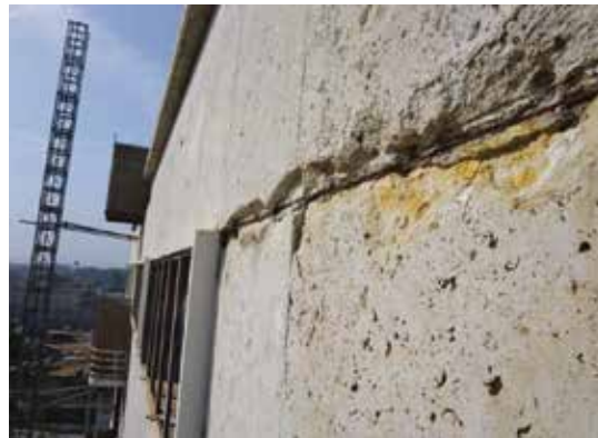
Limestone panel edges located along corroded steel shelf angles were spalling and cracking.
