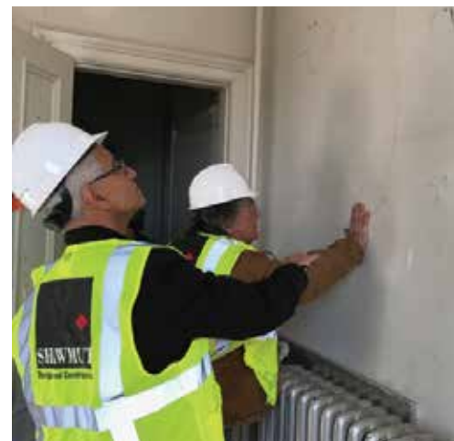
Figure 6. Investigating post-move cracks.
