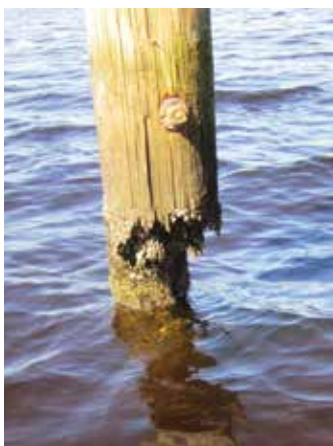
Figure 2. Wood pile deterioration near waterline.
