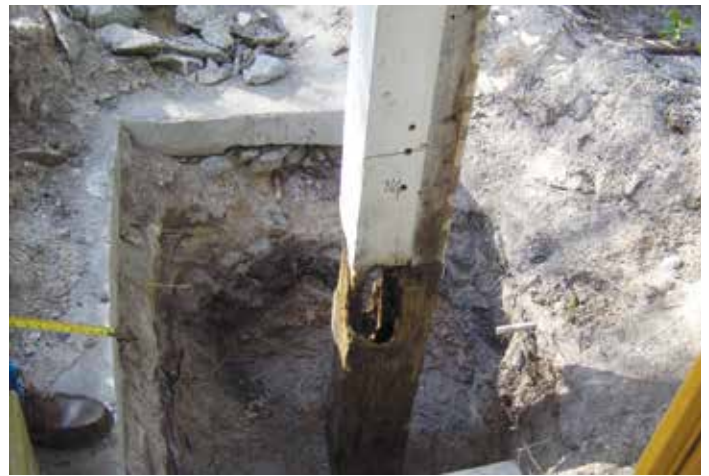
Figure 1. Wood pile deterioration near grade.
