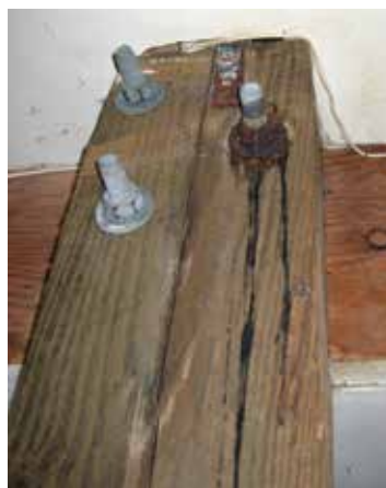
Figure 3. Corrosion of bolt due to wicking at the top of an interior pile under a coastal home.
