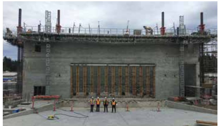
Elevation of the CMS wall and beam during construction. Approximately 40 feet of 60 feet completed.
