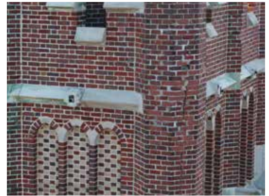
Figure 3. Drone head-on close-up image of deteriorated masonry.
