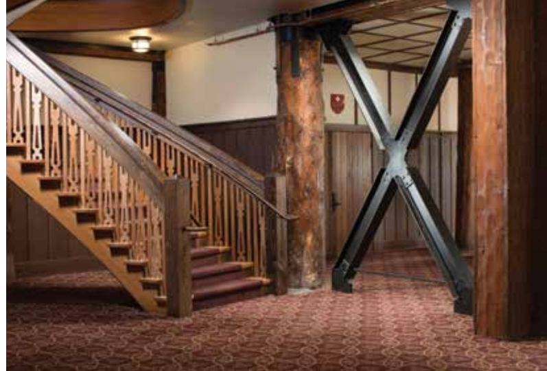
Braced frame in the basement level of the lobby. Courtesy of Mark Bryant Photographics.
