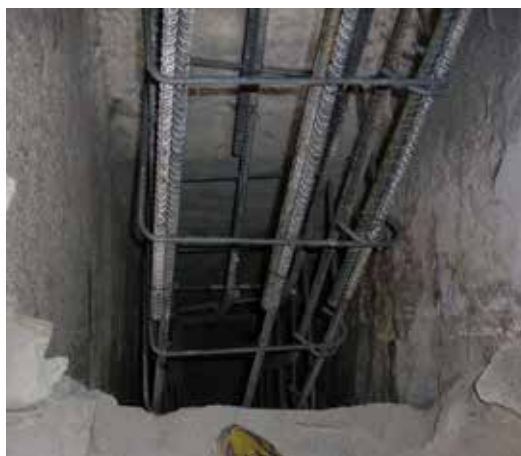
Reinforcing cage inserted into the full-height flue of the dining room chimney. Courtesy of Dan Cooke, JVA, Inc.
