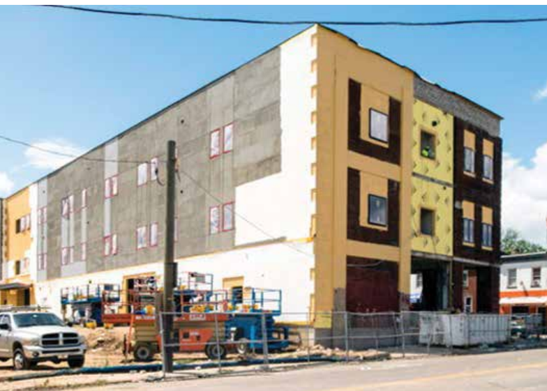
Figure 14. Lateral capacity of the post-renovation three-story building was assumed adequate based on the theory that the original six-story building sail area and mass translated to larger wind and seismic loads.
