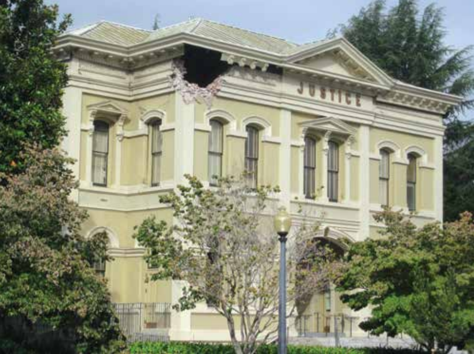
Figure 1. Entry showing damage taken the morning of the earthquake.
