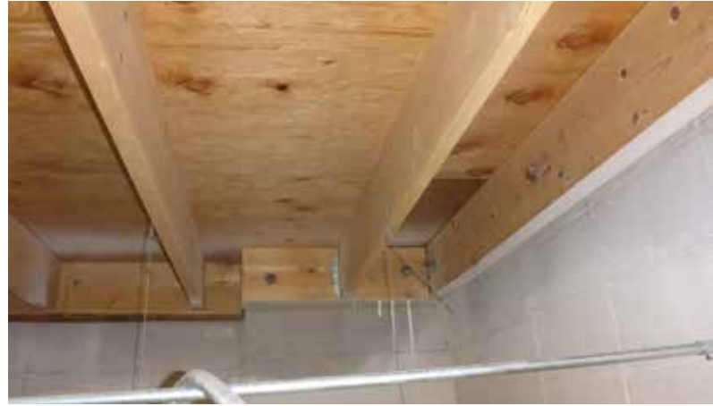
Figure 1. Wood diaphragm connections and shear walls not visible from the top surface of the diaphragm.
