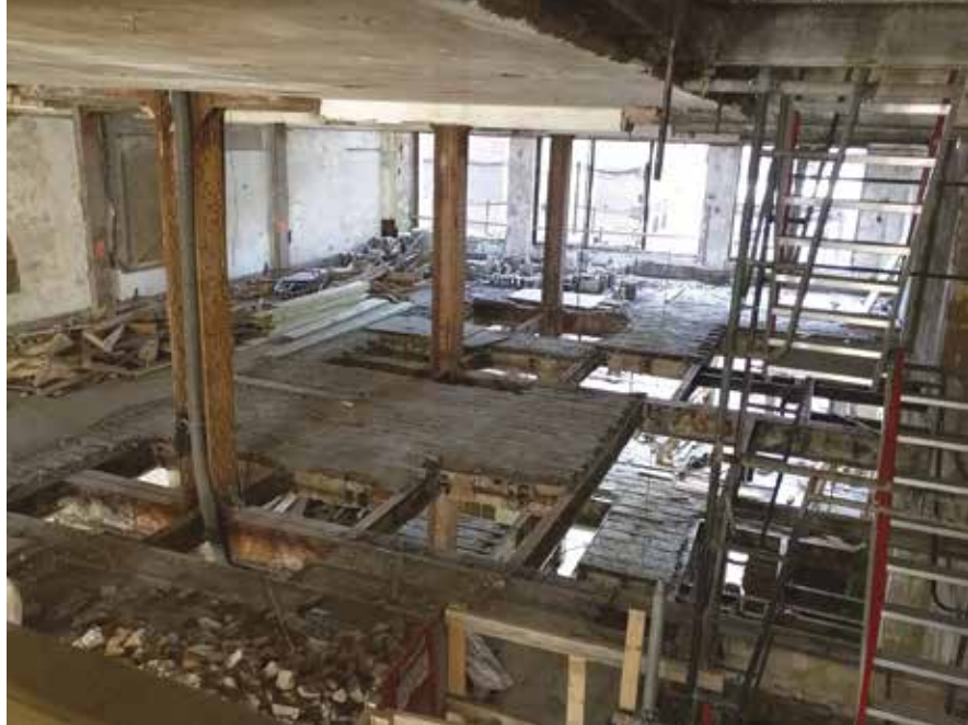
Figure 4. A typical level showing extensive demolition of the existing clay tile slab.
