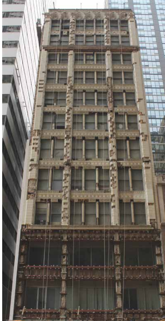
Figure 1. The exterior façade facing Michigan Avenue at the outset of the project.
