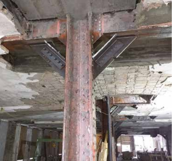
Figure 3. These double angle steel knee braces were installed at approximately 175 locations throughout the interior of the existing building.
