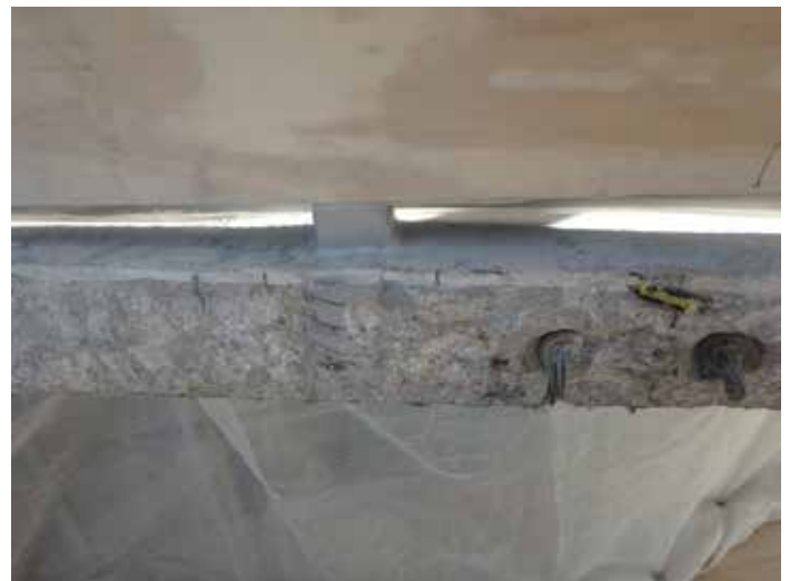
Figure 2. Concrete removal along a slab edge exposed grout pockets with missing hairpin anchor reinforcement.
