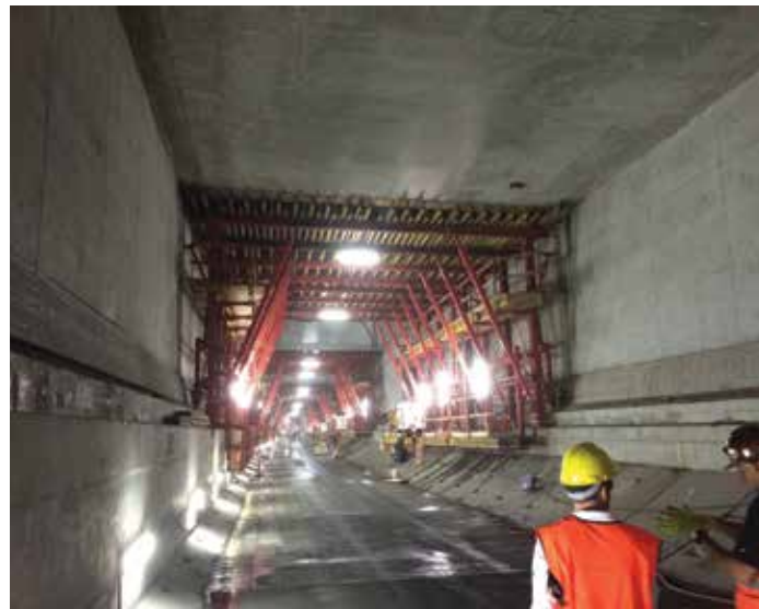
Final cast-in-place liner being installed within an initial, gasketed, pre-cast, concrete segmental liner.
