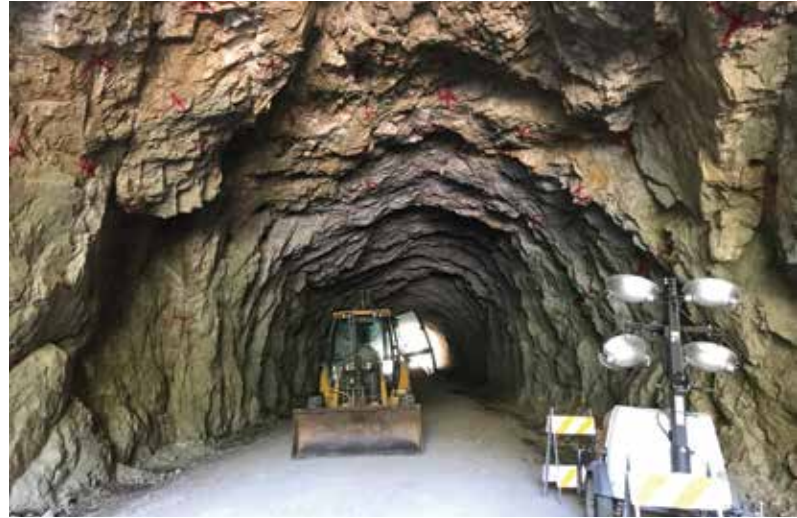
Unlined rock tunnel, subsequently supported with rock bolts and shotcrete to address rockfall risk.
