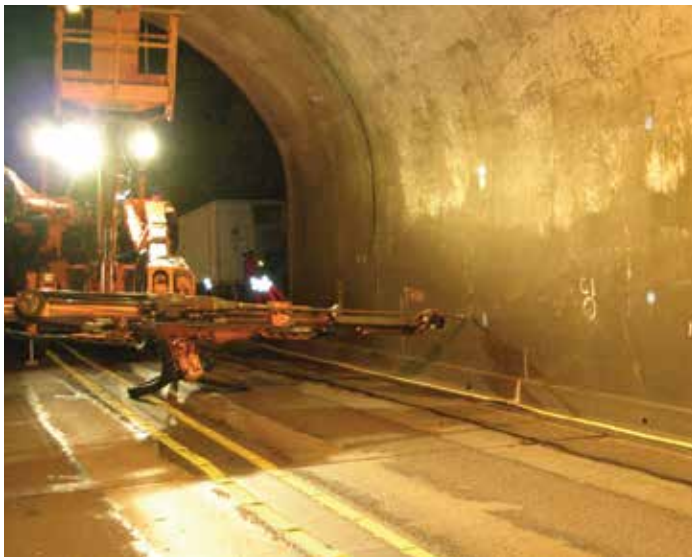
Drilling holes in an existing liner to fill with lightweight grout, for voids identified during the exploration program.
