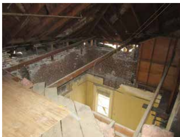
Figure 2. Courtroom view from the attic where brick partially collapsed the ceiling below.
