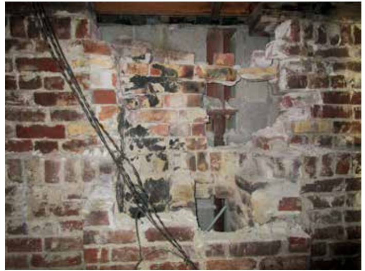
Figure 4. Partially collapse of URM wall due to adjacent Administrative Annex Framing.
