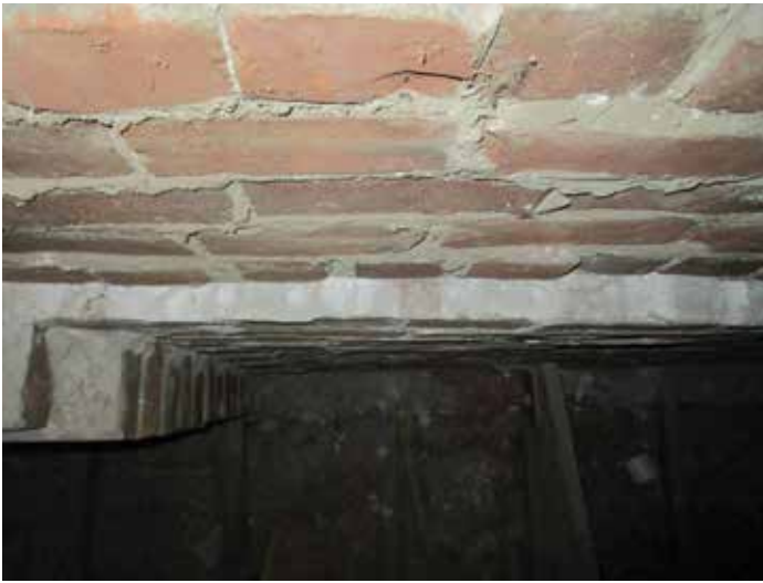
Figure 3. Horizontal offset of brick in the attic.
