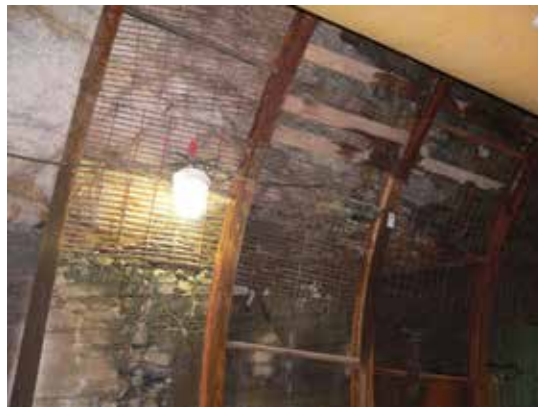
Figure 2. Shear zone in rock tunnel excavation.
