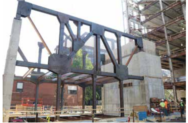
Construction progress elevation view of long span, steel story truss with steel hangers down to the first-floor structure.
