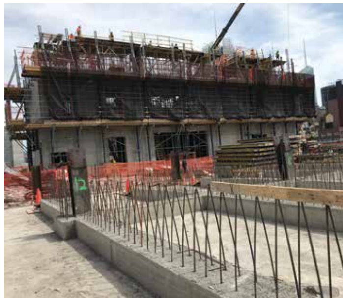
Figure 6. Reinforced concrete core emerging above the roof slab of the existing building.
