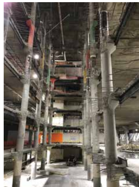
Figure 7. Shoring-free slab demolition for the core with temporary steel above the slab and permanent steel below the slab.
