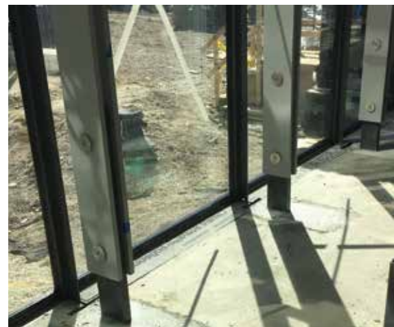
View of the erected steel paired plate mullions and two-bolt connection at the base of the glass wall.
