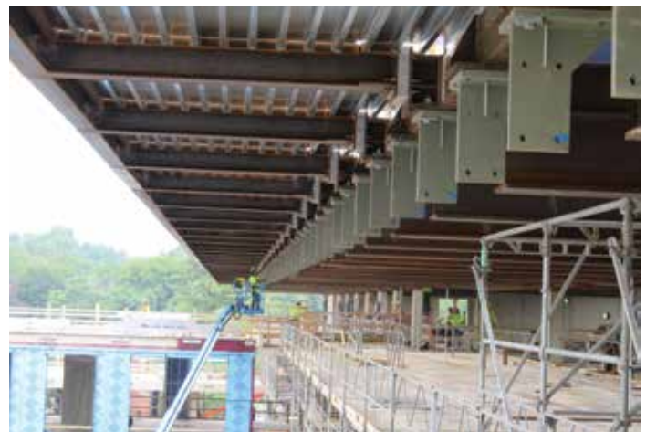
View of the erected roof framing and curtain wall connection plates at the top of the wall.
