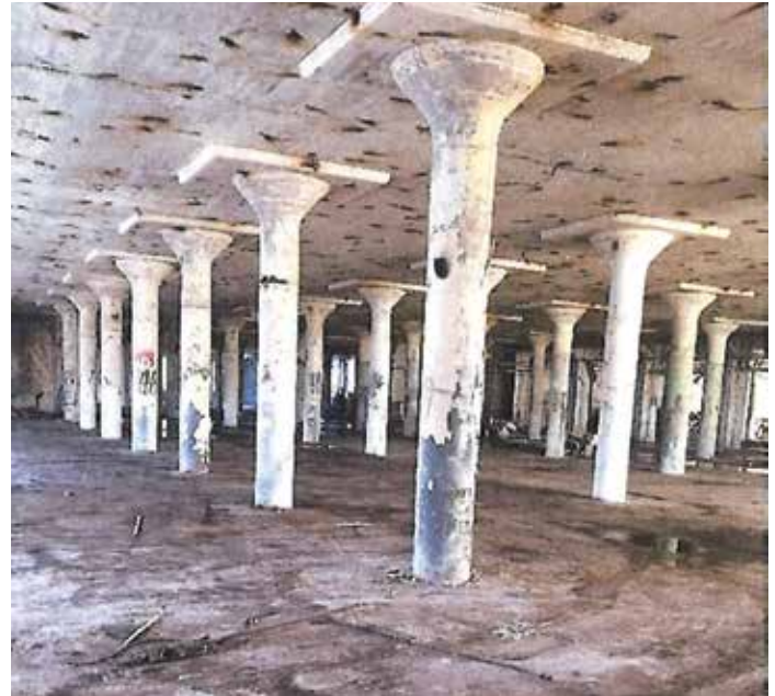
Figure 4. The 6-story structure was constructed as a reinforced concrete, flat slab supported by round and rectangular columns with column capitals and drop panels.
