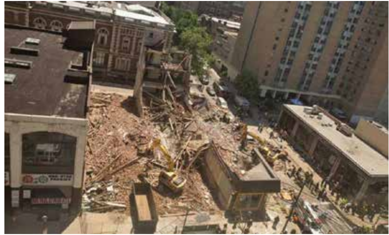
Figure 1. The aftermath of a June 5, 2013, building collapse associated with demolition of a series of adjoining two- and four-story mercantile loft structures onto the immediately adjacent, one-story Salvation Army Thrift Store building in Philadelphia. Courtesy of Lindsay Lazarski, WHYY.
