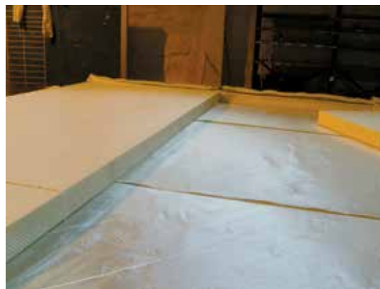
Fiberglass fabric is rolled out into the molding tool in the required direction, and a Fiber-reinforced foam core is placed before vacuum infusion.
