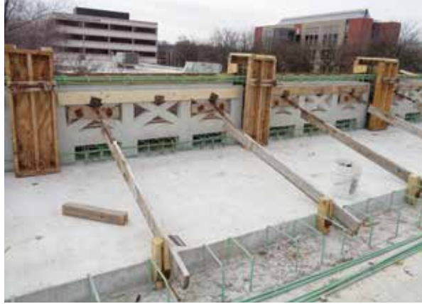
During construction, the reticulated balustrades used a combination of precast and cast-in-place elements to allow for utilities and to produce complicated concrete details to a high quality.
