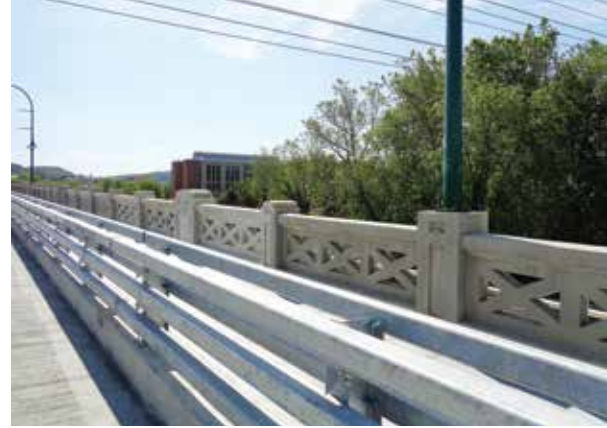
A new crashworthy barrier at the curb allows for reticulated balustrades and sidewalks narrowed from 11 feet to 7 feet to allow for adequate geometrics for bridge inspections.
