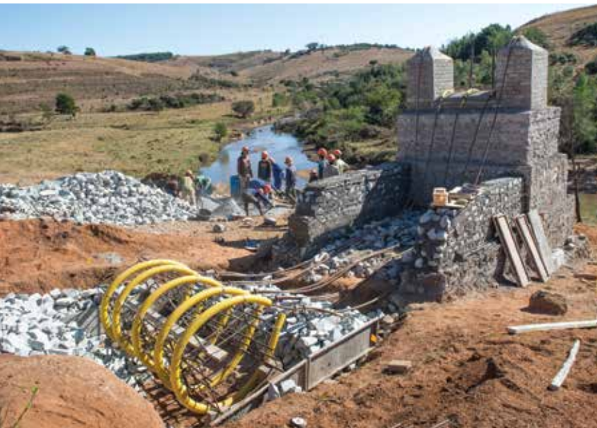
Preparing to pour an anchor after completion of towers. Courtesy of Madison Sankovitz.
