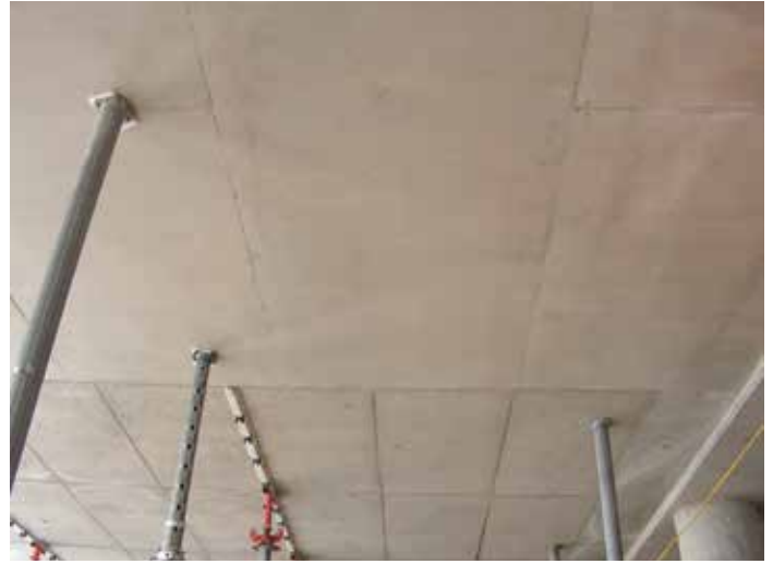
Architectural concrete is protected during the reshore phase to prevent inadvertent damage.
