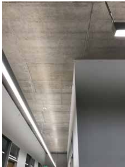
Completed slab soffit in lab corridor; the surface is formed with HDO plywood. Courtesy of Payette.
