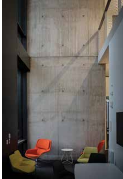
View of walls in study lounge with aligned formwork and tie holes. Courtesy of Payette.
