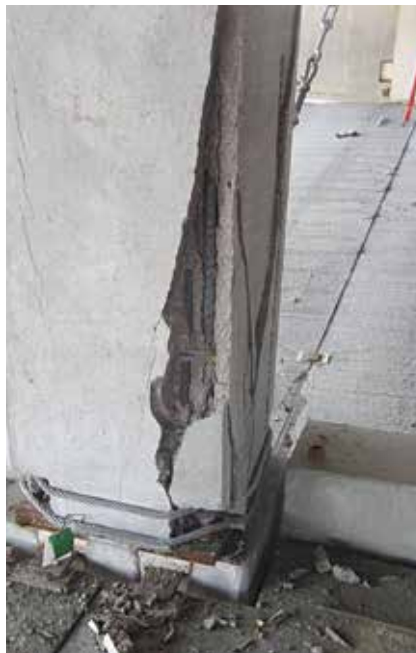
Figure 5. Local failure of the precast column due to lack of grout.
