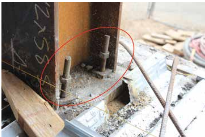
Figure 2. Protruding anchor rods after shim stack punched into pilaster below the column.
