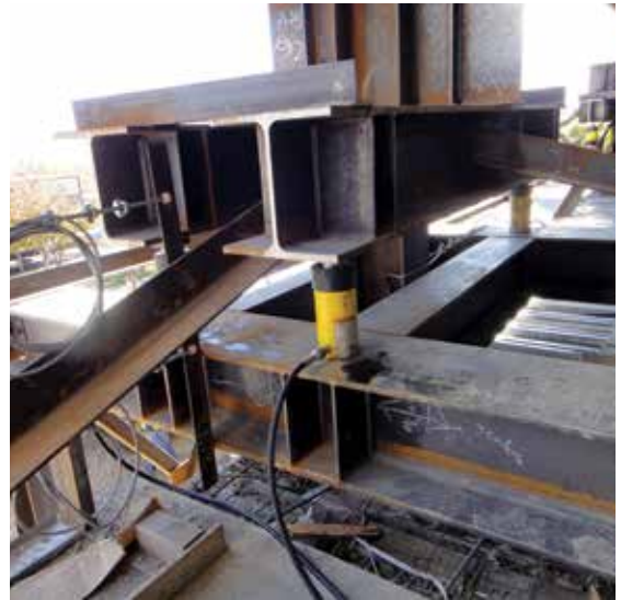
Figure 4. Apparatus to lift building frame to the proper position following failure.
