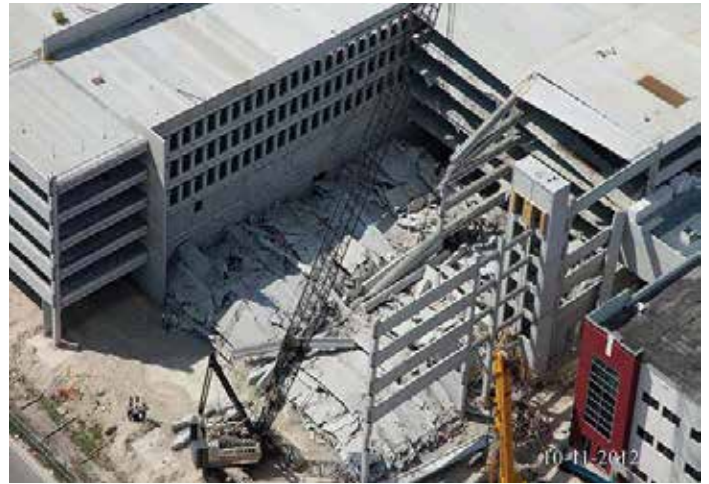
Figure 1. Aerial view of the Miami parking structure collapse. Courtesy of OSHA.
