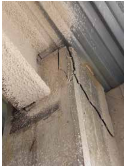
Figure 3. Failure of pilaster viewed from below.
