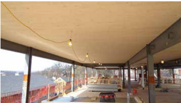
CLT floor structure to be exposed as a ceiling in the residence hall.
