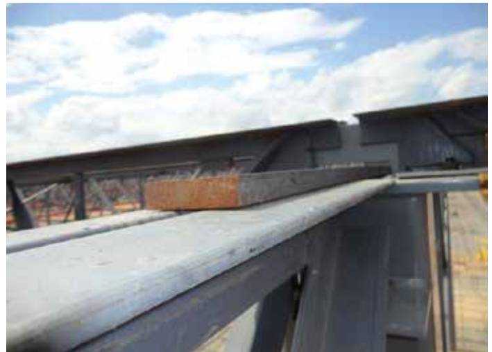
Figure 2. Joist girder moment connections to the strong axis of wide flange columns. Courtesy of Johnson & Burkholder, Engineers.
