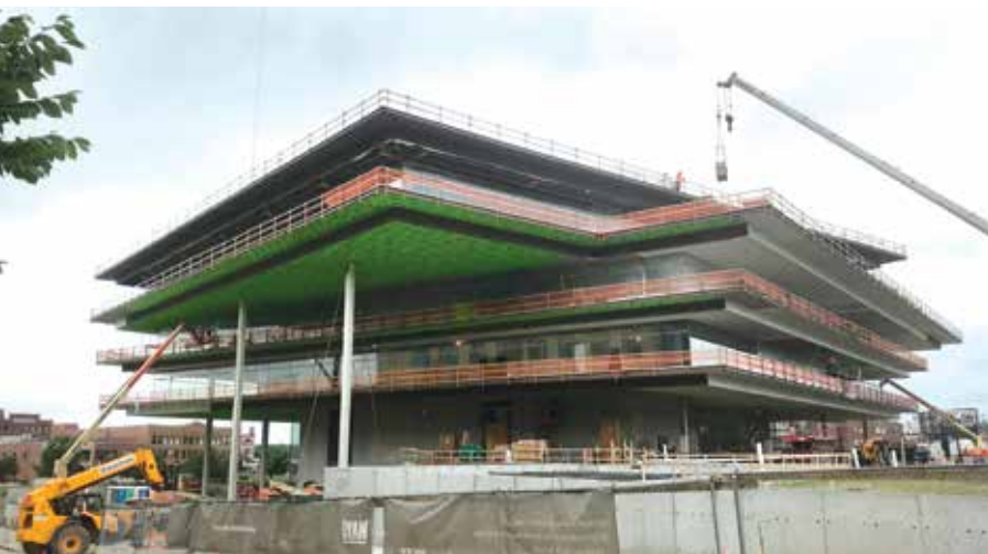
Figure 2. The northeast exterior face of the building during construction (note super columns are supporting 5 th and 6 th floor).
