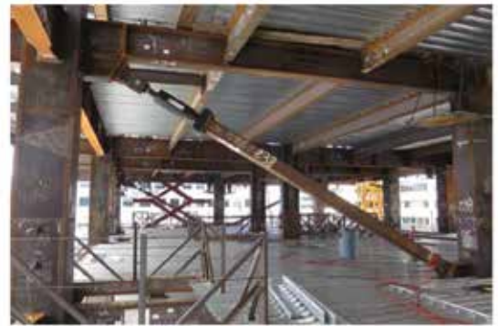
Typical Installed VDD & Extended Brace
