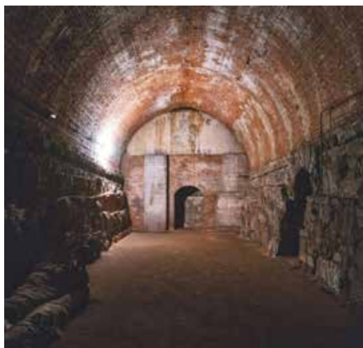
Arch block interior with vault transverse and longitudinal symmetrical and asymmetrical through-cracks, revealing various forces acting on the load bearing structure.
