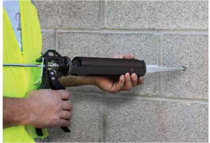
Injecting adhesive into drilled holes in masonry to make an anchor connection.
