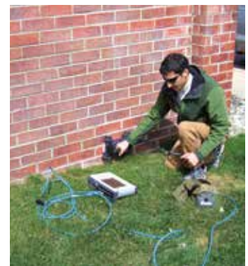
Figure 6. Surface-penetrating radar equipment in use to locate reinforcement and grout in clay masonry construction.
