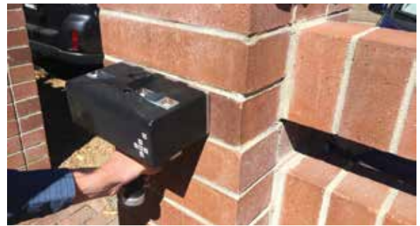
Figure 4. Ultrasonic imaging equipment used here to determine solidity of a reinforced clay masonry column.
