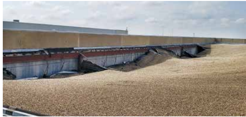
Rain collapse at an FM Global insured location in the southern United States.
