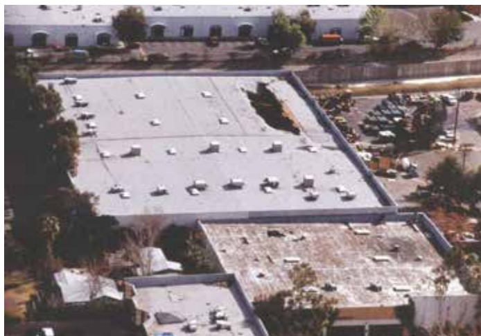
Figure 2. Diaphragm failure due to inadequate continuous crossties for wall anchorage. Courtesy of Doc Nghiem.
