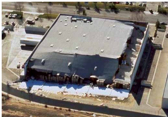
Figure 3. Damage to tiltup concrete building due to loss of wall anchorage during the 1994 Northridge earthquake. Courtesy of EERI.
