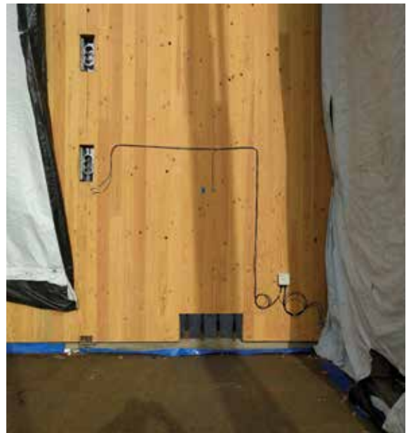
Moisture monitoring equipment – part of the "Living Lab @ Peavy Hall" study at OSU – installed on a shear wall at the George W. Peavy Hall construction site.
