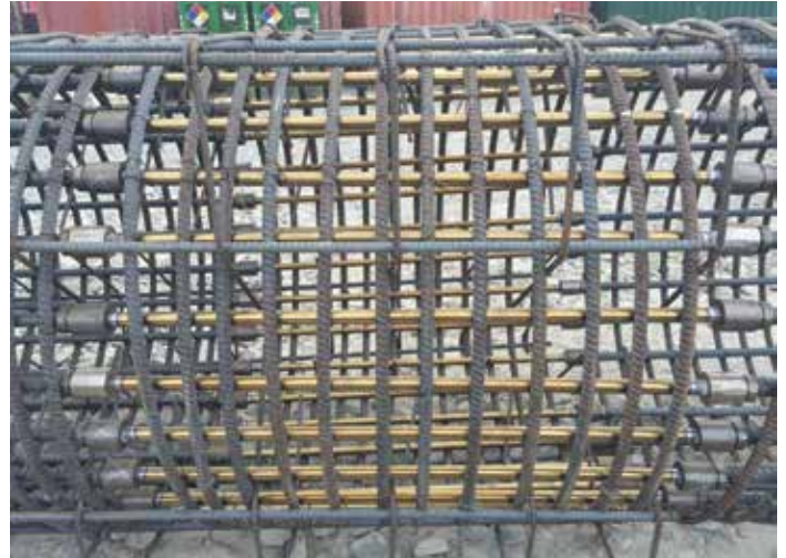
A column cage ready for erection with SMA bars spliced in the plastic hinge region.
