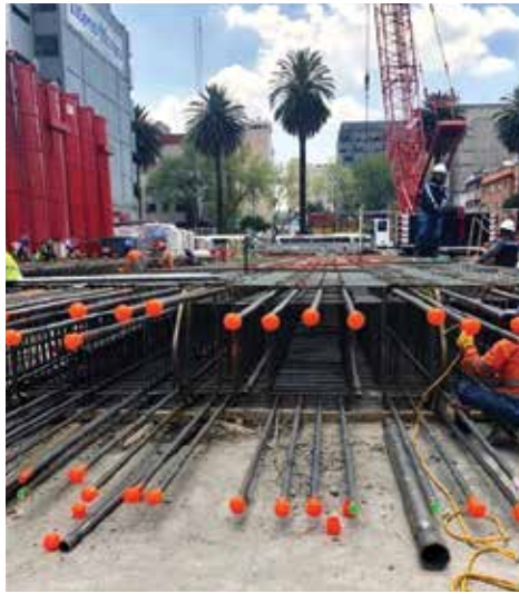
Figure 10. Reinforcement of a typical barrette from a recent high-rise project in Mexico City that has a length of 40 meters (130 feet).
