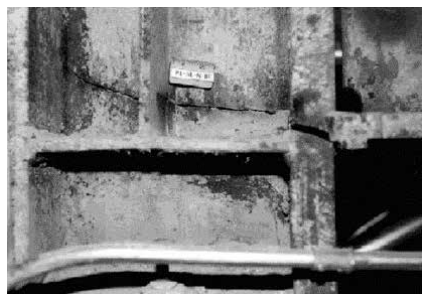
Figure 4. Fracture extending from CJP weld across column web.
