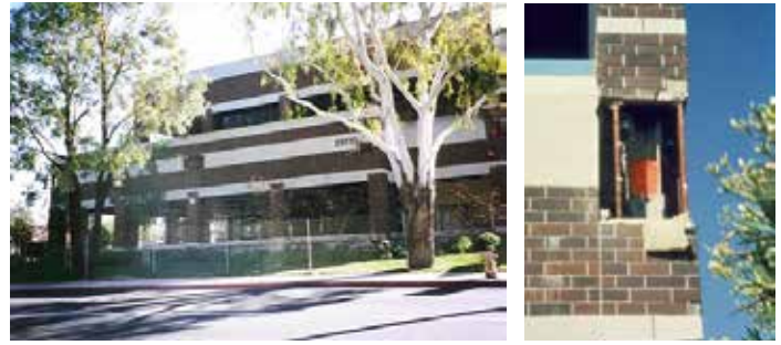
Figure 3. The Southern California Automobile Association Building. To the right, a large permanent drift in the building.
