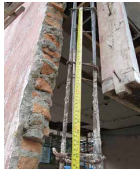
Typical inadequate reinforcing in damaged school buildings.
