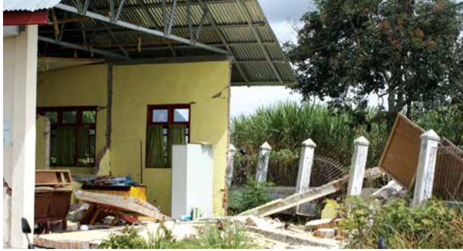
Collapse of gable end wall in a classroom building. Courtesy of Educational Department Aceh Tengah.
