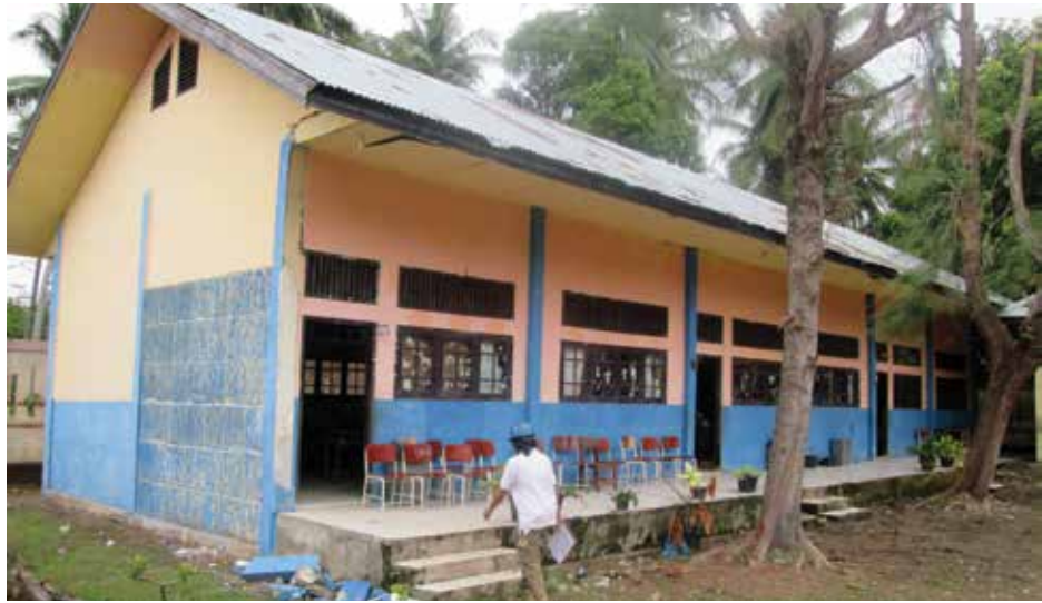
Typical classroom building – Note the lack of confining elements at door and window jambs, lack of ring beam at the side wall, and very minimal length of wall pier in the longitudinal direction.
