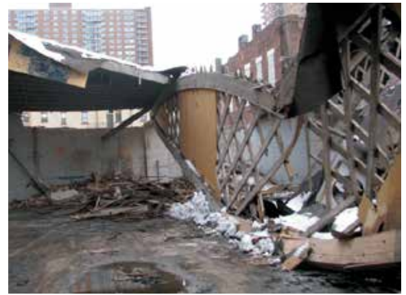
Figure 5. Collapsed “Belfast” bowstring truss. Wood failed at bottom chord mid-span. Note relatively small snow cover.
