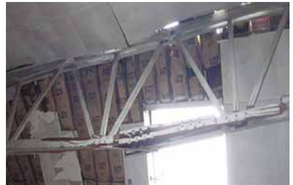
Figure 6. Bowstring truss failed at connection.
