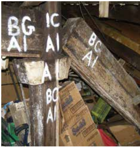
Figure 2. Failure of connection and collapse of timber girder supporting first floor.
