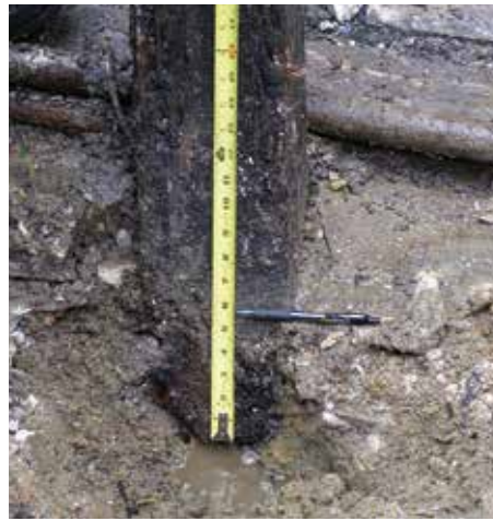
Figure 3. Rotten base of timber post.
