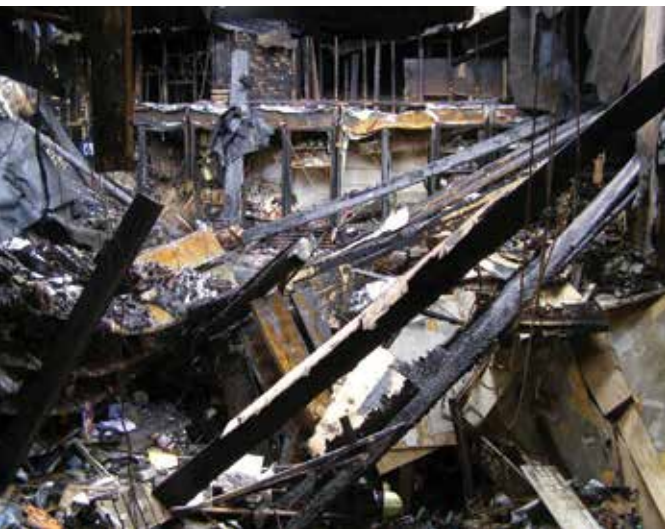
Figure 1. Debris field – roof charred joists cover collapsed first floor.
