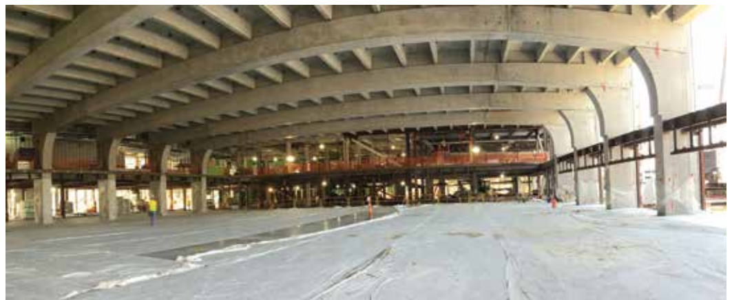
Figure 4. Long-span concrete flooring system under construction, showing precast double tees placed on a precast bent. Courtesy CannonDesign, Inc.
