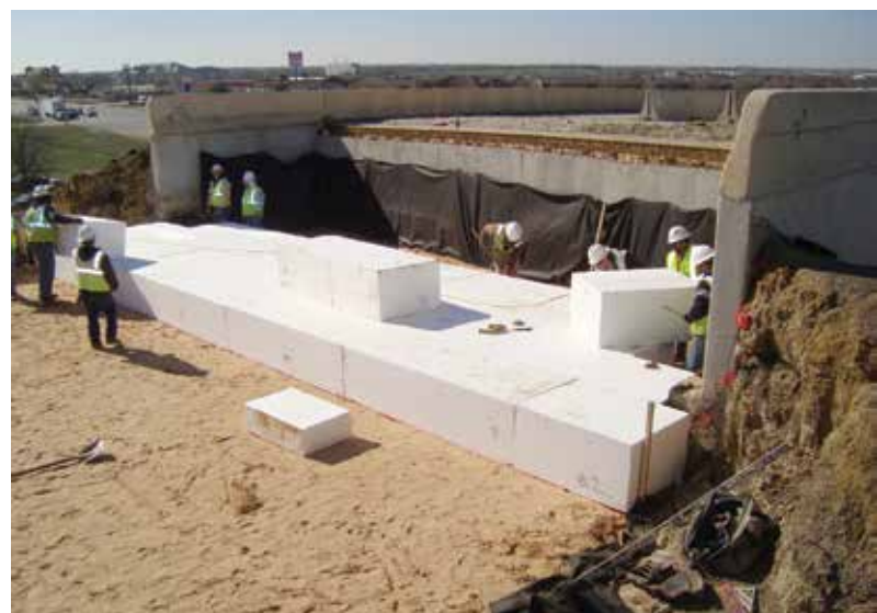
Lightweight, yet incredibly strong, the geofoam blocks are moved into position by laborers while engineers assure the stack configuration is built as specified.
