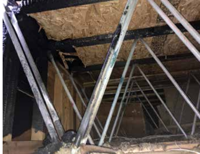
Figure 5. Damaged top chords of the hybrid truss.
