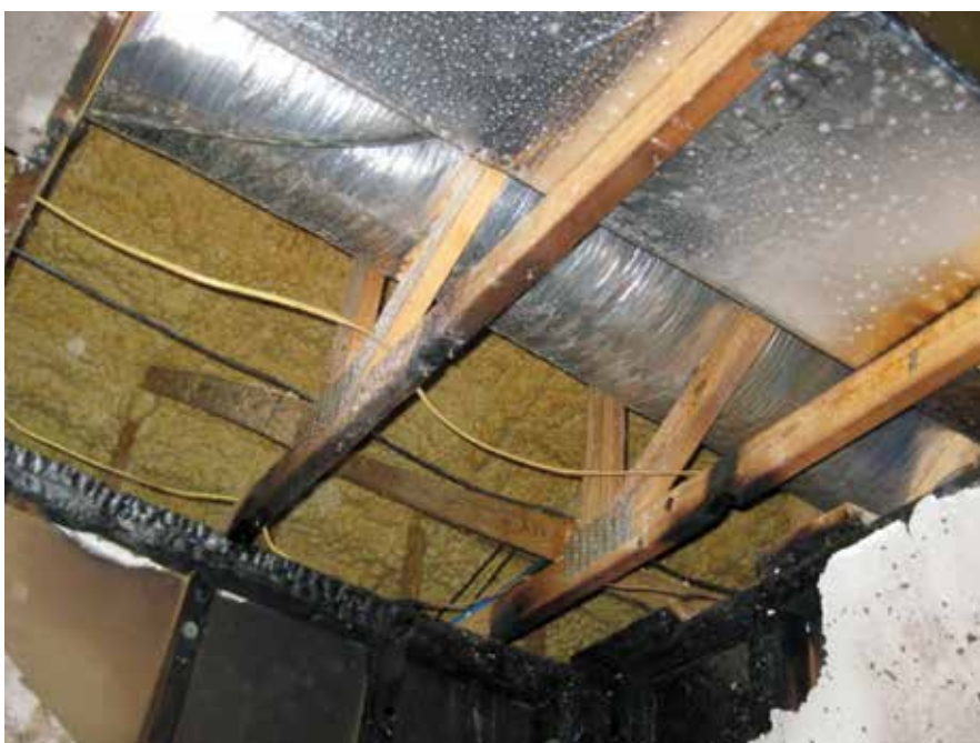
Figure 1. Charred bottom chord truss members.
