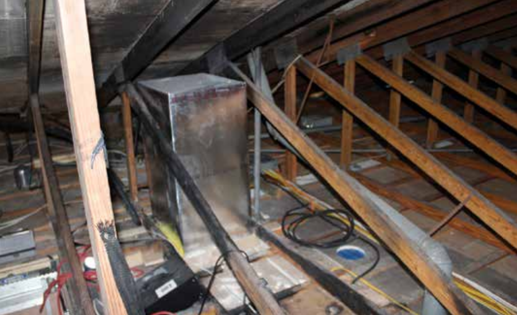
Figure 3. Damaged truss members and the HVAC plenum.
