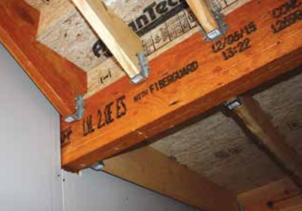
Figure 2. Stair landing beam shaft wall structural penetration prior to fire caulk installation.
