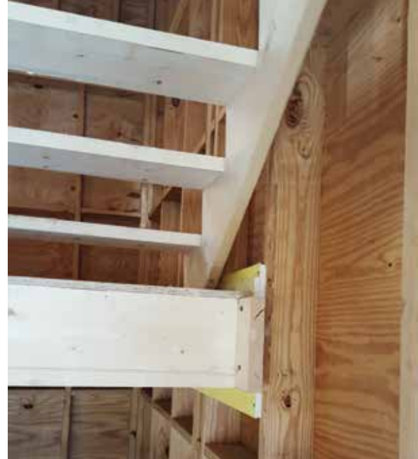
Figure 2. Stair landing framing attached to shaft wall through two layers of gypsum.
