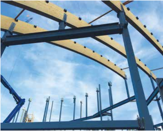
8¾- x 36-inch glulam roof beams were erected onto a steel infrastructure; steel columns were tilted toward the center of the building at the large spans to accommodate lateral spreading.
