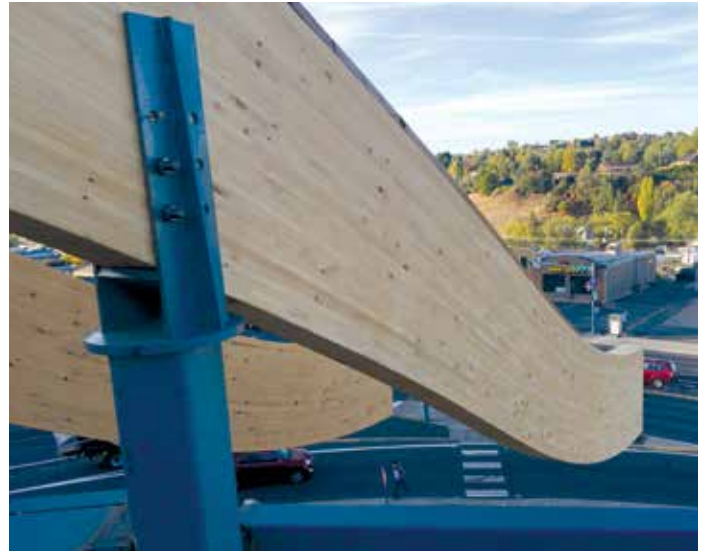
Double curvature glulam beams were seated onto the steel column pedestals using round capital plates to showcase the structural steel column-to-glulam beam connections.
