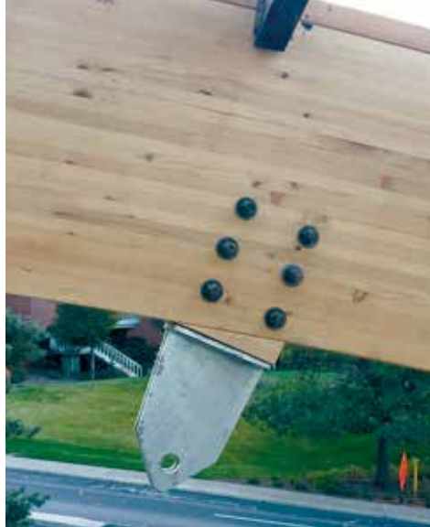
This single curvature beam was connected to a turned double-tapered glulam column using a kerfed connection to hide the connector's side plates from view.
