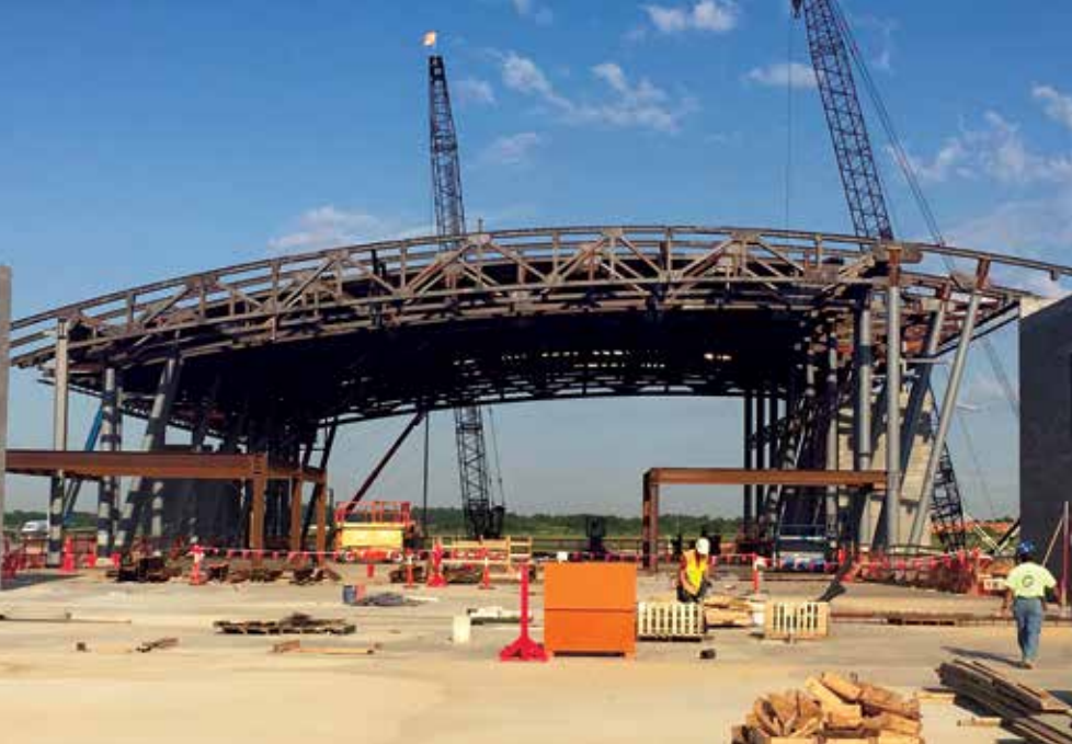
Erection of arched steel trusses spanning the width of concourse over the elevated concrete slab.
