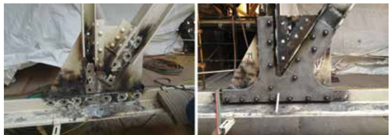
Figure 3. Truss node with truss members welded to gusset plate and rivets removed (left) and reinforced with new finger gusset plates and high strength bolts (right).
