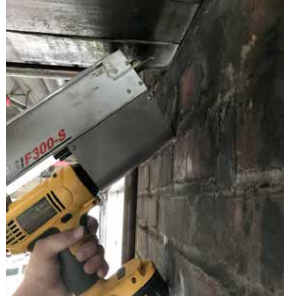
Figure 2. Resistograph test to determine the extent of deterioration at the bearing end of a bowstring truss embedded in masonry.
