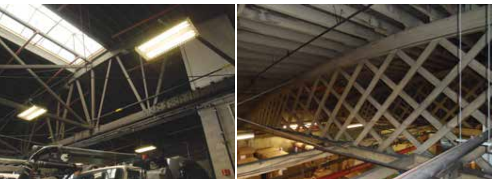
Figure 1. Bowstring trusses in which web elements are discrete (left) and are a lattice system (right).
