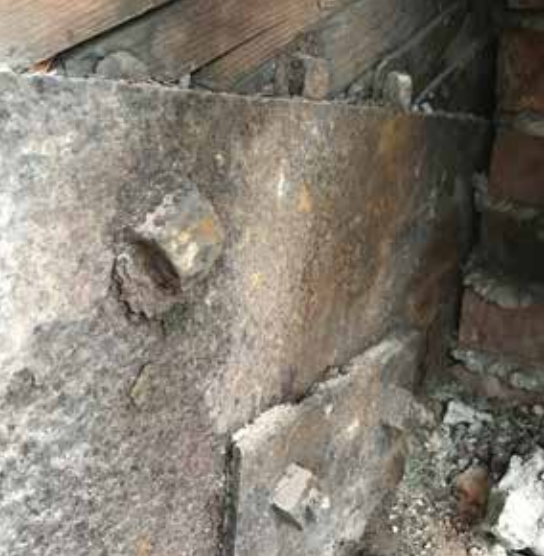
Figure 3. Exploratory probe opening at the bearing end of a bowstring truss embedded in masonry.
