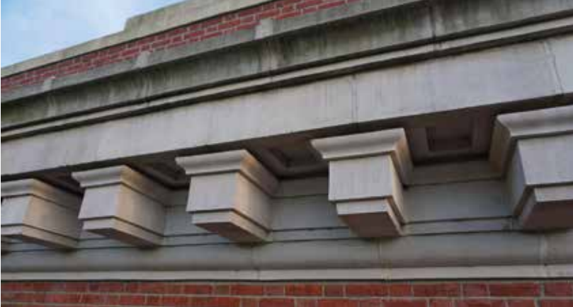
Figure 2. Terra cotta cornice spot replacement with ICCP in 2004. Two pieces of terra cotta were replaced on the full cornice, and the entire steel outrigger system is protected by Impressed Current Cathodic Protection.
