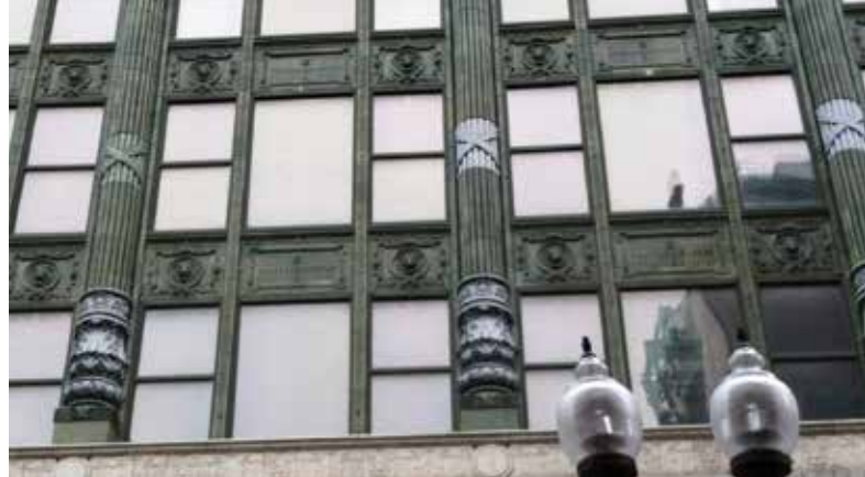
Figure 3. Discoloration of GFRC units used in conjunction with original terra cotta.
