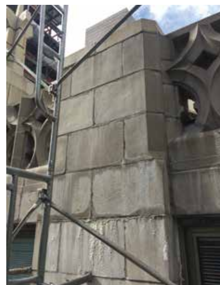
Figure 6. Full wall replacement cast stone units. Note the shrinkage, water infiltration, and leaching.
